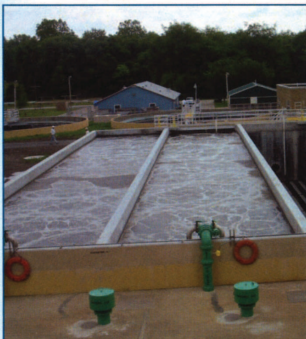
Secondary aeration at the facility was expanded to fully treat a 22 MGD peak wet weather flow.
