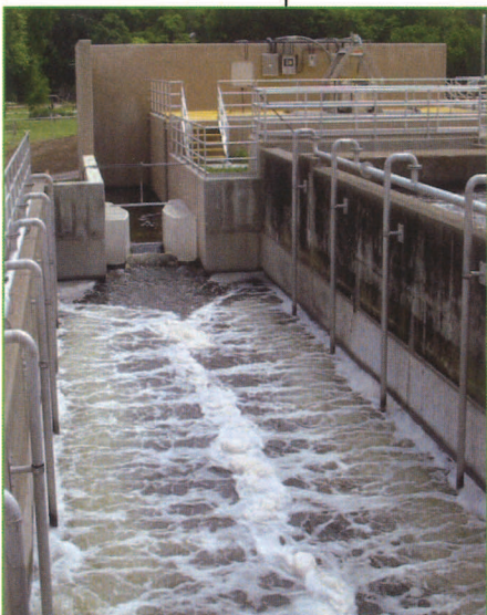
Treated effluent is re-aerated to make sure the aquatic life in the Wabash River is protected.
