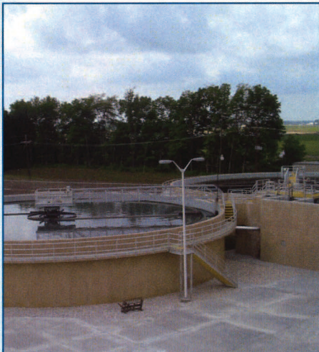
The two new primary clarifiers each handle a peak flow of 11 MGD.
